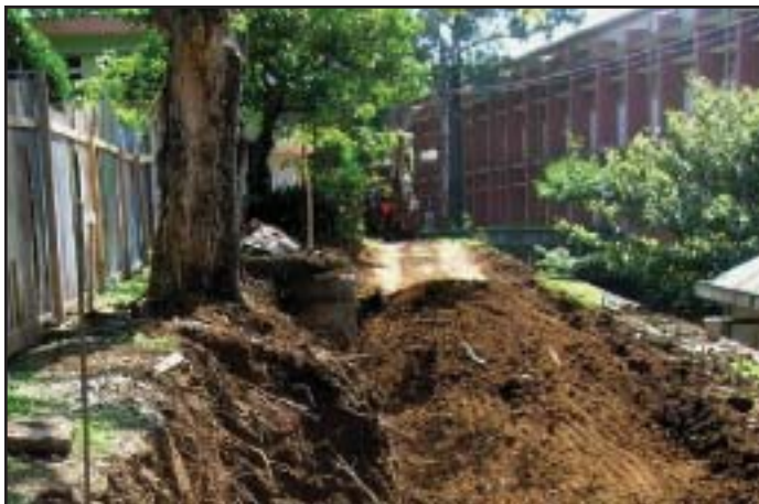
Figure 1. Root depth varies by site. At the construction site pictured here (University of Costa Rica; San José, Costa Rica), nearby trees root systems can be seen to penetrate several meters deep.
